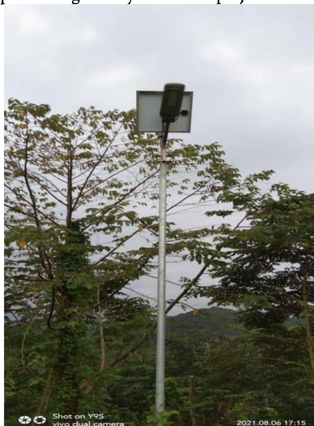
Figure 5 : Photograph showing solar system in the project area
